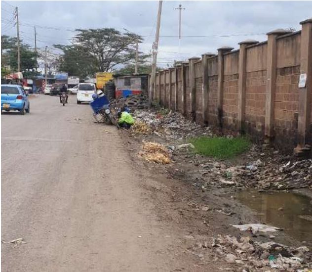
Clogged open drainage channel in Mlolongo Central area
